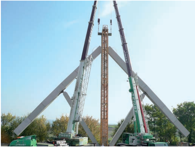
Fig. 16. Lowering the top points of the bridge girders with the help of mobile cranes
