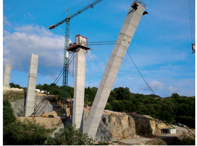
Fig. 4. Arnoia Bridge in Spain built using the method of lowering arches (photo credit: VSL Heavy Lifting , Switzerland)
